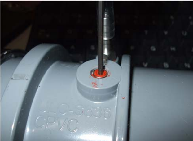
Figure 3 - Cross Section of ECO Installed on Top of Flue Assembly Bracket and Set Screw
